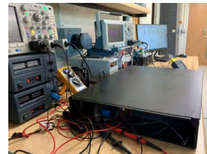
Online UPS inside a chassis for testing under practical conditions of a data center. Photo provided.
